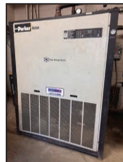
PARKER AIRTEK CESM100-A4-F1 REFRIGERATED AIR DRYER
