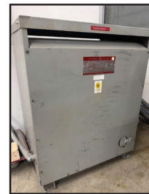
GENERAL ELECTRIC 112.5 KVA DRY-TYPE QL TRANSFORMER
