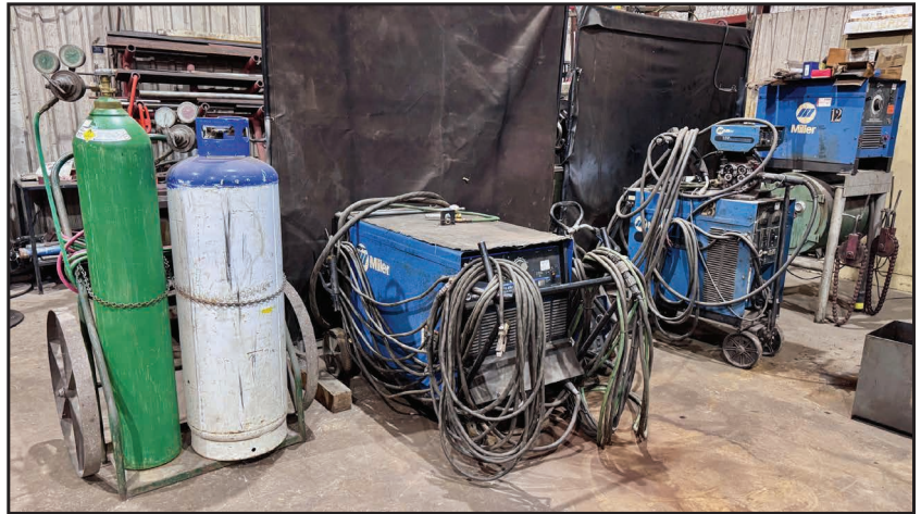
ASSORTED WELDING EQUIPMENT
