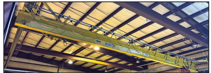
DELTA 6-TON SINGLE GIRDER BRIDGE CRANE
