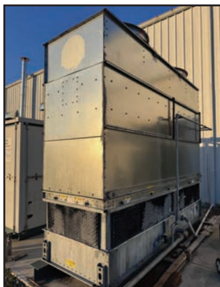
M&M CARNOT PURE CHILL 62TR CHILLER SYSTEM
