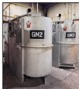
VIEW OF LINDBERG 16-RO-1500-A3 ELECTRIC ATMOSPHERIC GENERATORS
