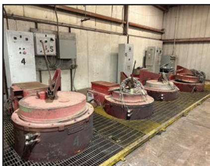
VIEW OF LINDBERG TEMPERING FURNACES
