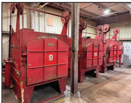
VIEW OF LINDBERG BOX FURNACES
