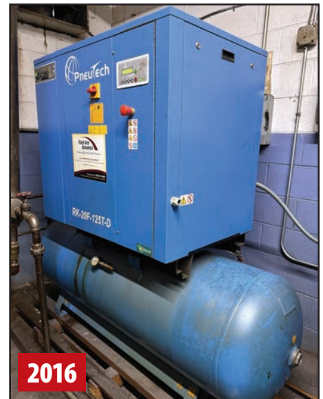
2016 PNEUTECH 20 HP AIR COMPRESSOR
