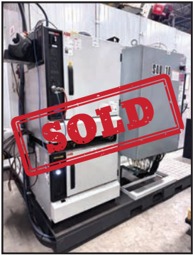
VIEW OF ABB IRC5 ROBOT CONTROLS
