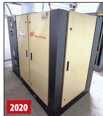
2020 INGERSOLL RAND RS37I 50 HP VARI-SPEED AIR COMPRESSOR
