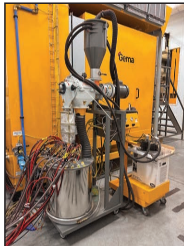
GEMA RECLAIM SYSTEM
