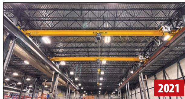
2021 FRONTENAC 40' X 200' FREE-STANDING CRANE SYSTEM
