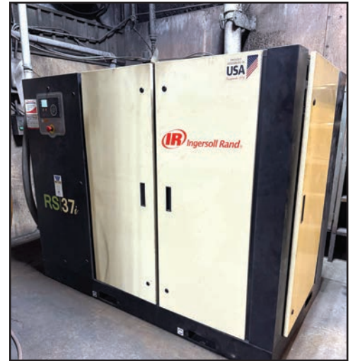
INGERSOLL RAND RS371I 50 HP AIR COMPRESSOR
